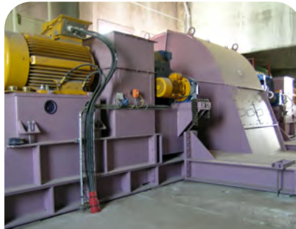
High capacity elevator head (1600 m 3 /h, height 65 m, 2x200 kW)
